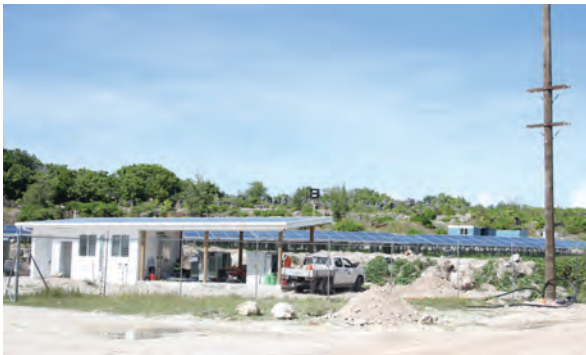
New Zealand MFAT/ European Union 1.1 MW Solar Farm
