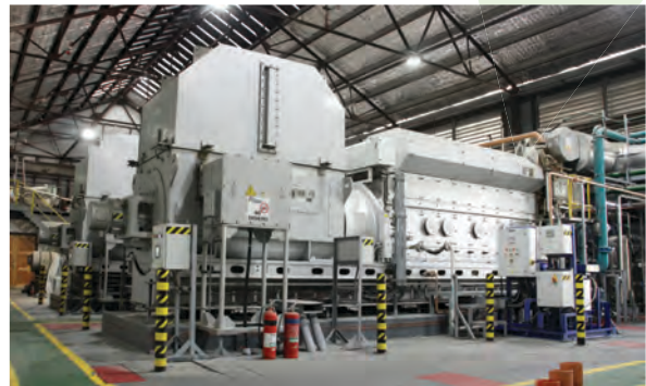
2.85 MW MAN Diesel Engines
